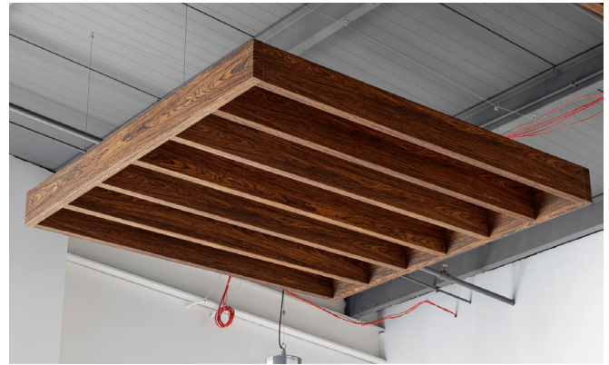
For the cafeteria, we created a custom-tailored beam configuration to simplify the installation process by reducing the number of pick points needed in the ceiling.
